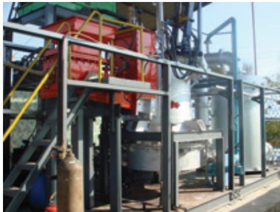
Figure 3: PTDR-100 system commissioned to process a wide range of solid waste streams, including medical waste, industrial process waste (organic and inorganic) and pharmaceutical industry waste
